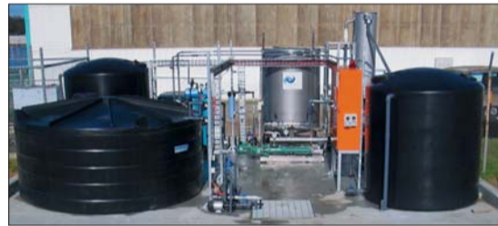
Acqua Environmental Australia's comprehensive, fully automated bilge and wastewater treatment facility on Bullock Island...
